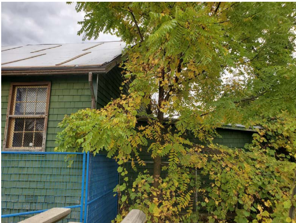
Figure 15: Former Canteen Building, northeast façade, northwest façade, and northwest addition (looking southwest)
