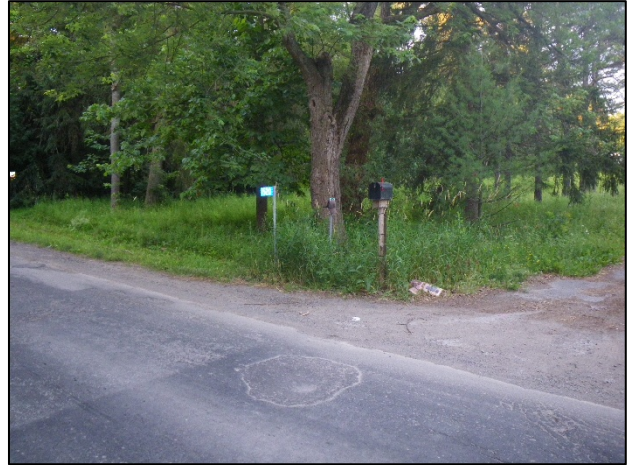
Facing southwest across road toward downstream end of culvert. Note lack of valley or floodplain.
