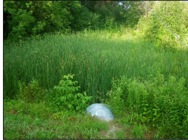
Upstream (west) end of culvert. Note no defined channel within a small cattail marsh.
