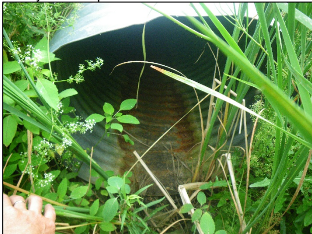
Upstream end of culvert facing downstream (northeast). Note dry conditions, lack of substrates within culvert, and lack of evidence of high flows.
