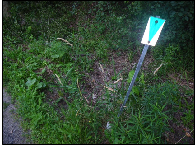
Upstream (east) end of culvert. Note no defined channel and terrestrial vegetation within roadside ditch.
