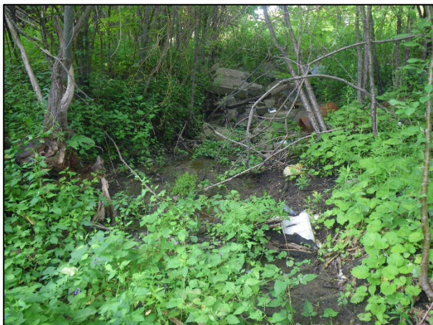
Downstream facing upstream (southwest) at downstream end of culvert. Note concrete debris and perched condition.
