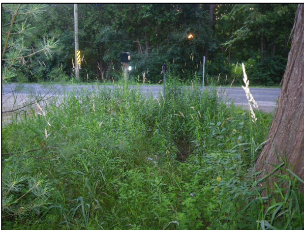
Downstream facing upstream (northeast) at downstream end of culvert. Note terrestrial vegetation.
