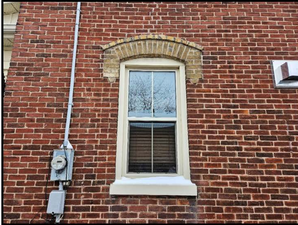
Image 15: Detail of Typical Window Opening of 442 King Street East (Photo taken on February 16, 2024; Facing West)
