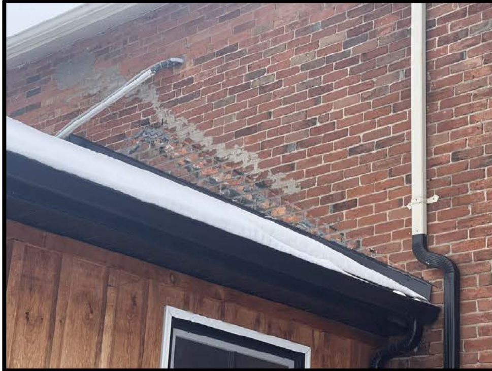
Image 17: Detail of Ghosting along Rear Elevation of 442 King Street East (Photo taken on February 16, 2024; Facing South)
