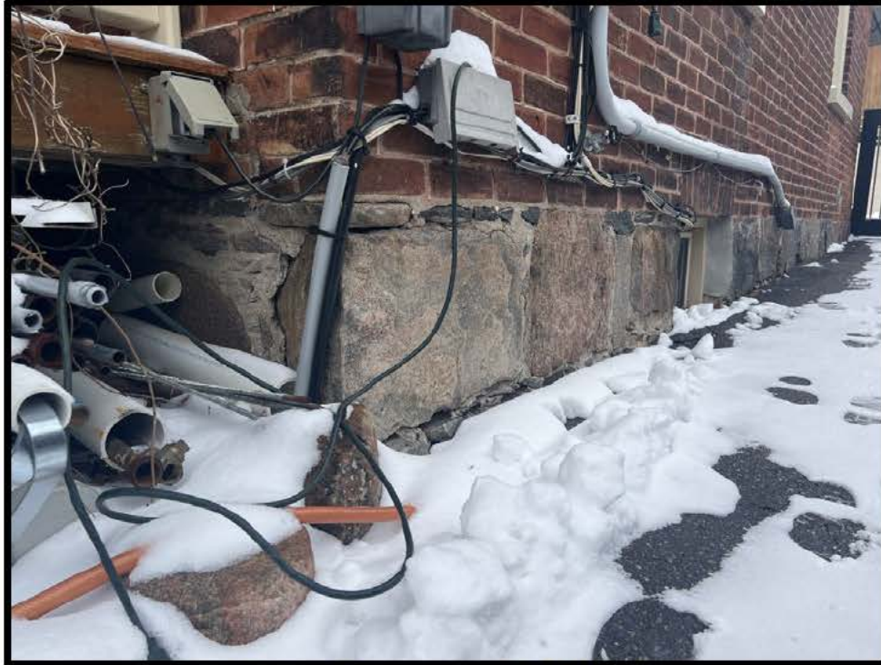
Image 13: Detail of Foundation of 442 King Street East (Photo taken on February 16, 2024; Facing North)
