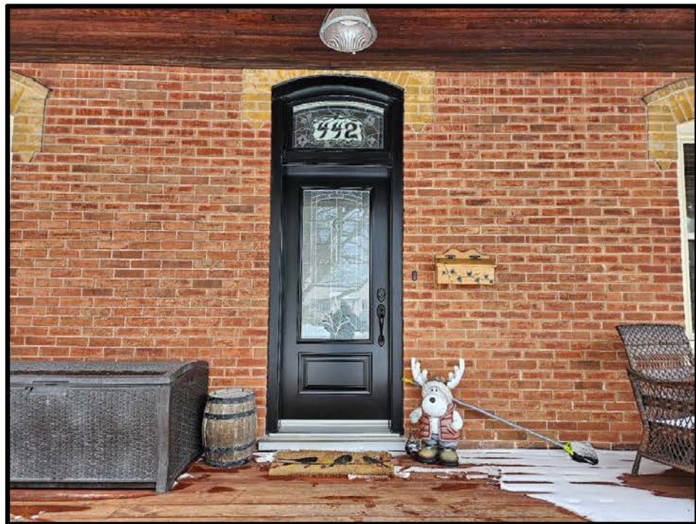
Image 10: Detail of Principal Entryway Opening of 442 King Street East (Photo taken February 16, 2024; Facing North)
