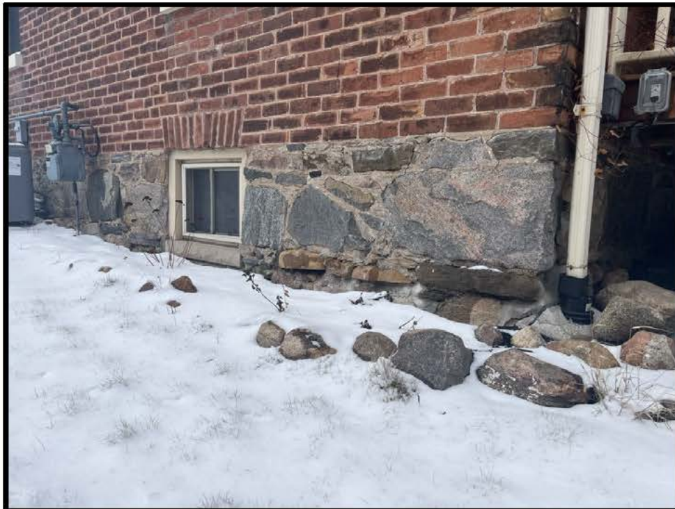
Image 14: Detail of Foundation of 442 King Street East (Photo taken on February 16, 2024; Facing Northeast)
