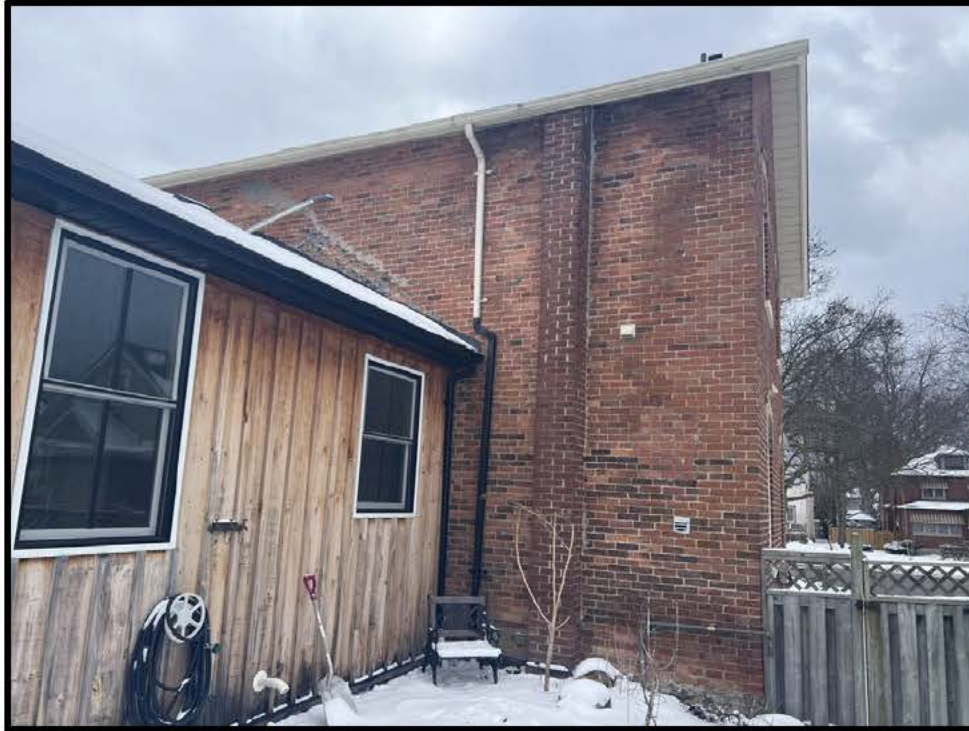
Image 5: North (Rear) Elevation of 442 King Street East (Photo taken on February 16, 2024; Facing South)
